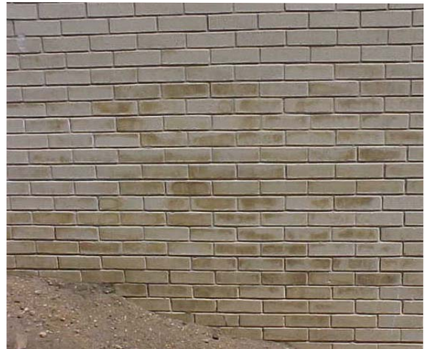
Photo 7 Yellow Vanadium Stain
