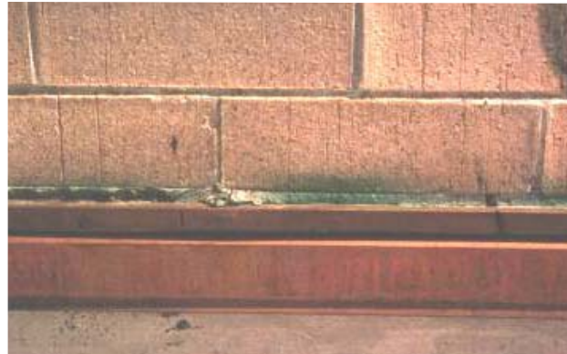
Photo 12 Stain from Copper
