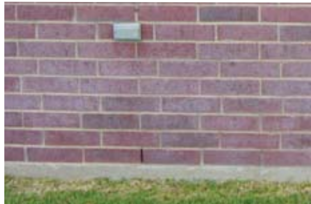
Photo 14 Hard Water Stain
