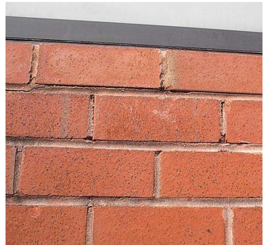
Photo 1 Mortar Joints in Need of Repointing
